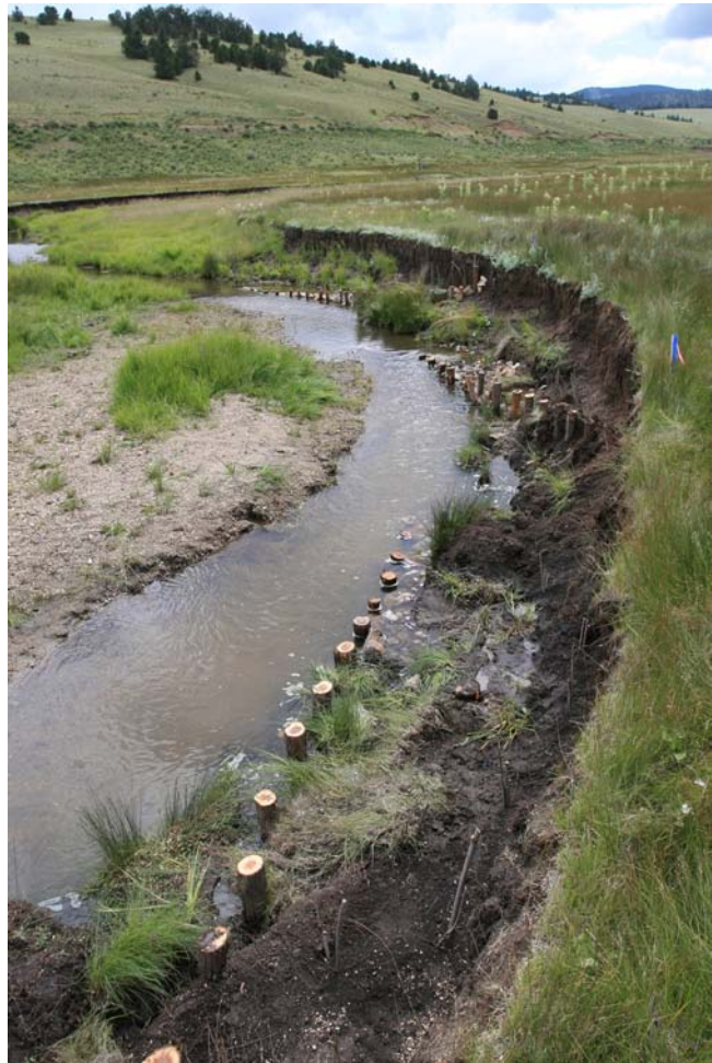
Three post vane structures help heal the creek by moving the water flow away from eroding banks on the outside bend (note the willow cutting planted behind the vanes, which will help build a new bankfull bench). Photo by Courtney White
