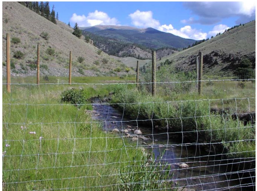
An herbivore exclosure under construction, one of fifty built since the mid-1990s to protect native vegetation along Comanche Creek. Photo by Bill Zeedyck
