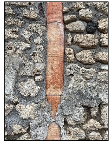
Ceramic pipe in a wall
